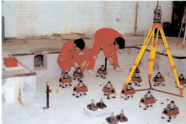
Positioning the BW-Fixators using a co-ordinate system – steel wire attached to support brackets
